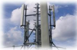
GSM Base Station
